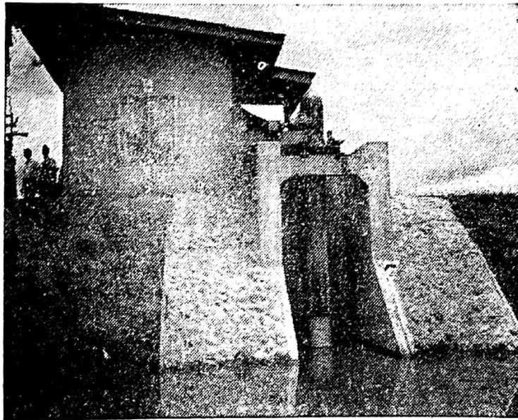
A low lift 16-inch pump installed in Sulipan, Apalit, Pampanga to irrigate 200 hectares.
