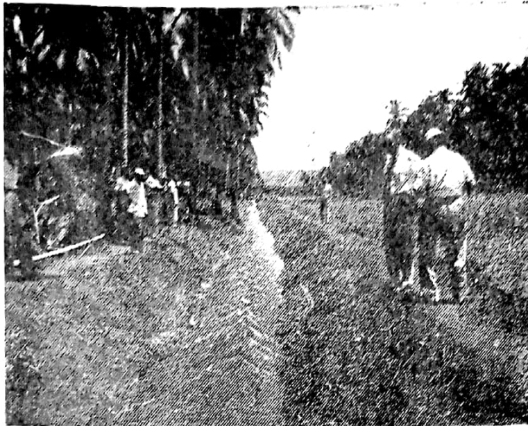
Irrigation water delivered by a 16-inch pump to irrigate 200 hectares in Sta. Cruz, Laguna.
